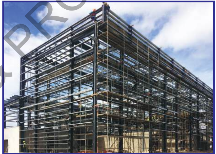
Fiji Airways Flight Simulator Centre Floor Area = 4000m 2 King Road, Martintar, Nadi.
