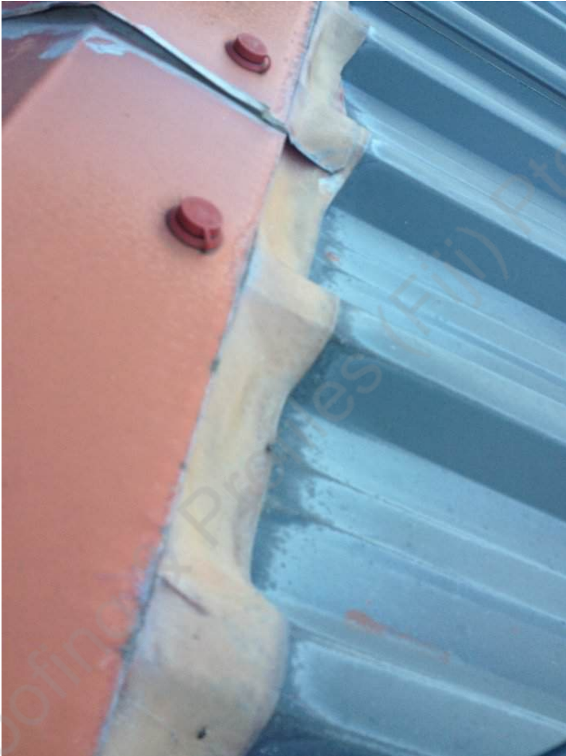
Lead in contact with coated or uncoated AZ will cause premature corrosion.
