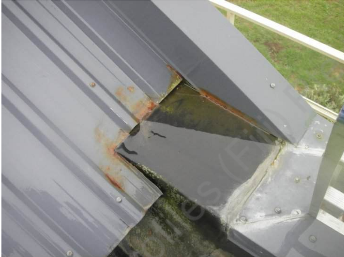
Butyl rubber in wet contact with coated aluminium and steel has been found to accelerate corrosion.
