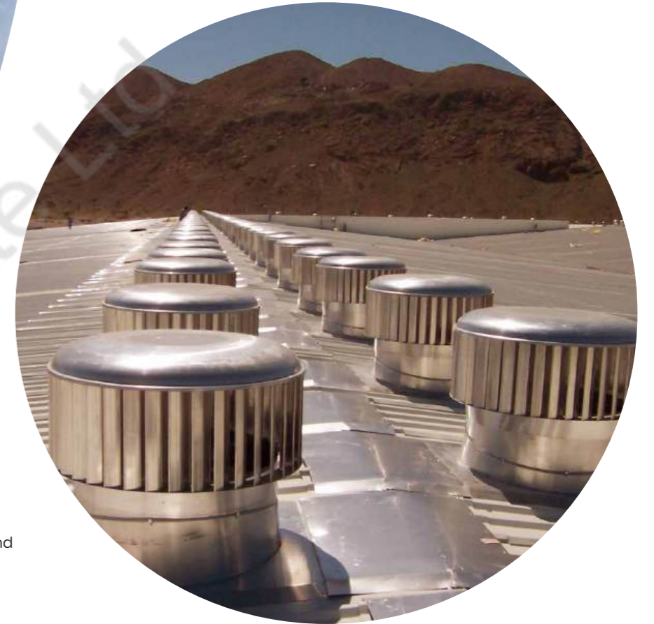
Toyota Spare Parts facility in Muscat Oman, Hurricane H900 for high ambient conditions >40°C.
