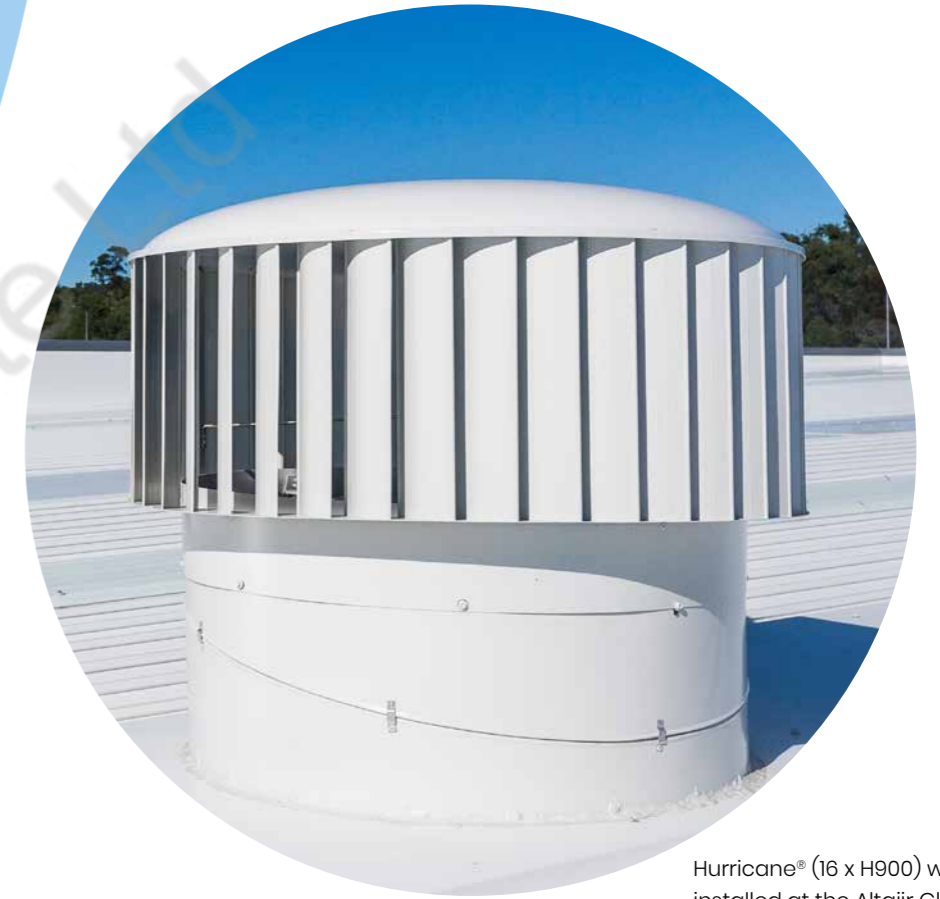
Hurricane® (24 x H800) was installed at the Brisbane Markets to reduce the level of moisture in the air.
