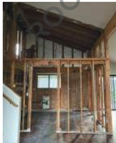
Before: Trescott's kitchen was incredibly dark, completely enclosed in walls and a suffocating, 7-foot ceiling.
