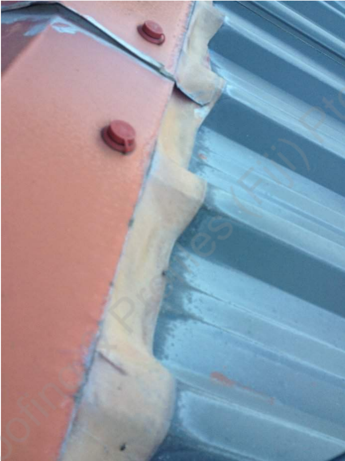
Lead in contact with coated or uncoated AZ will cause premature corrosion.
